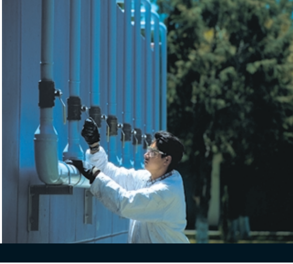
At the Sahagún facility, an employee regulates the air flow into the water treatment system basin.
